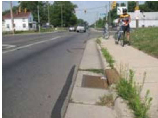
Roadway resurfacing should ensure that the transition between the asphalt and the gutter pan is flush, with no lip.
