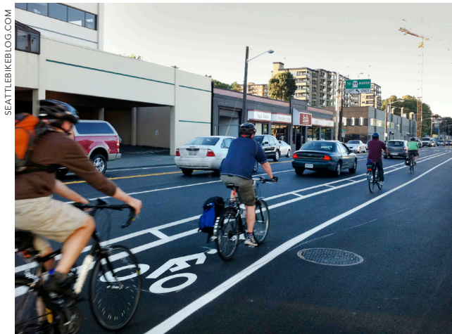
This buffered bicycle lane on Dexter Ave N offers increased space and more comfortable separation from moving vehicles than a conventional bicycle lane.
