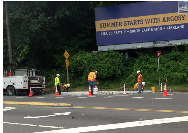
Installing a wheel curb to protect bicyclists in the bicycle lane from sharply turning traffic.
