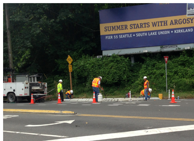
Installing a wheel curb to protect bicyclists in the bicycle lane from sharply turning traffic.
